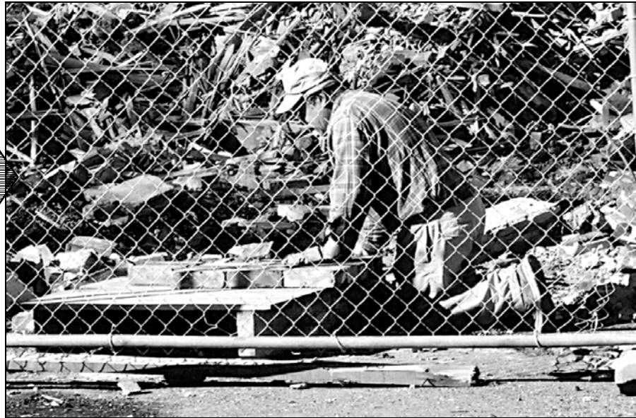
13.13. The brick cleaner begins to lay the first layer of a new pallet of bricks.
