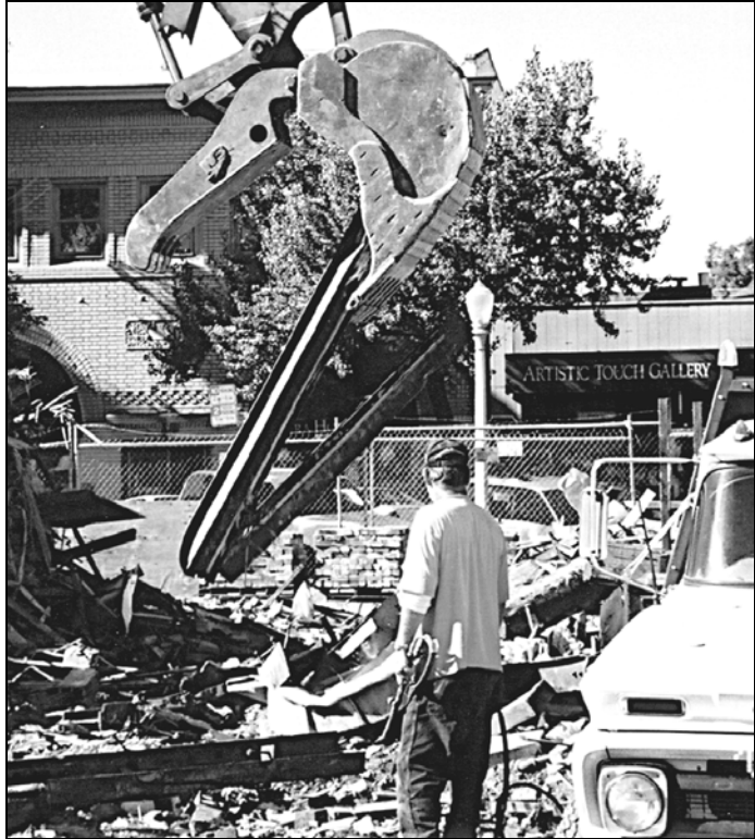
13.14. Bowers in the process of bending an I beam so that it will fit in the bed of a flat-bed truck.
