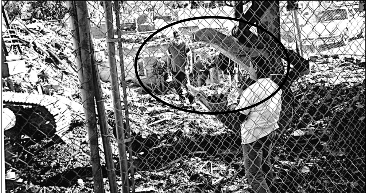
13. 18. A session of "throwing brick," Day 44 (October 31). The "claw" of the excavator is configured as a bucket into which the five people working the site are to "throw brick." The black oval shows Bowers and his helpers rummaging for brick at the basement level.
